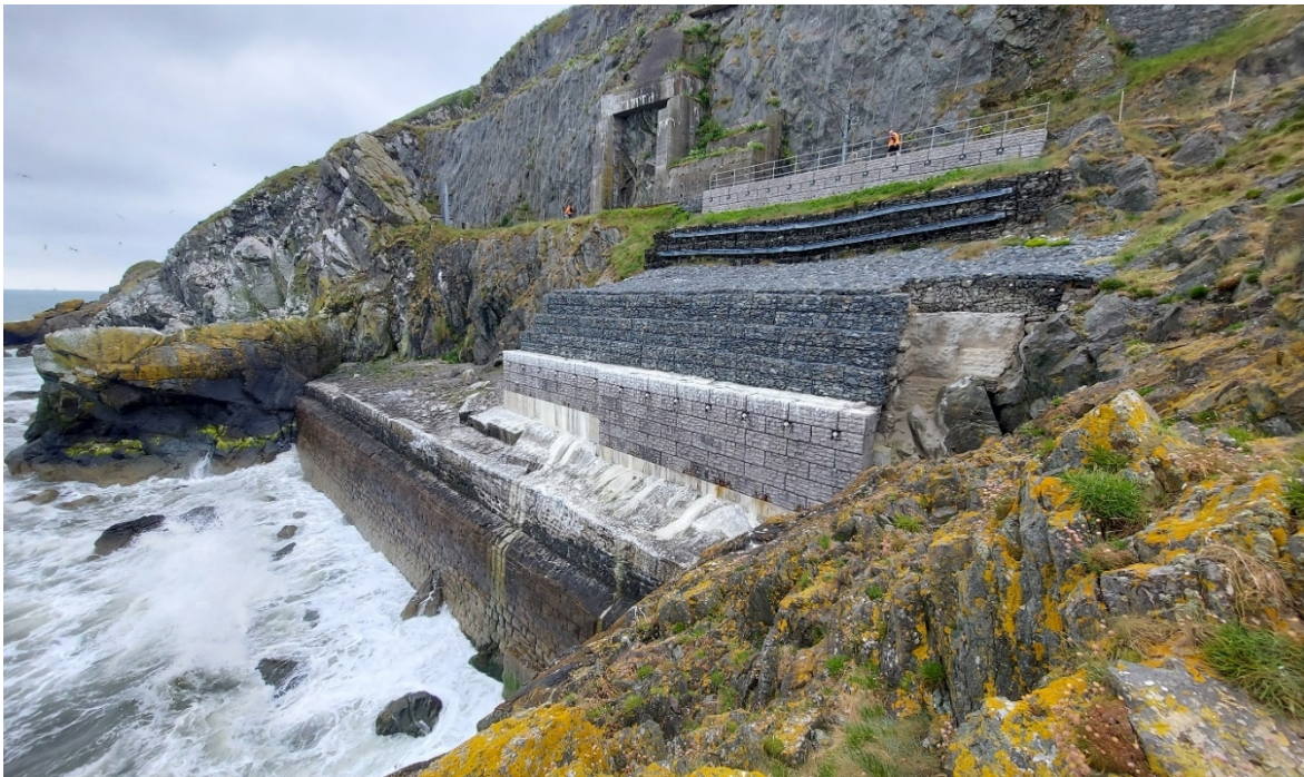
Figure 3 – CCA5-A: Another example of an engineered section can be seen here, located between two rock outcrops. The asset is made of a series of masonry walls, gabion baskets, rock anchors and concrete revetment which have been constructed at different stages. Again, rock netting is visible above the railway.
