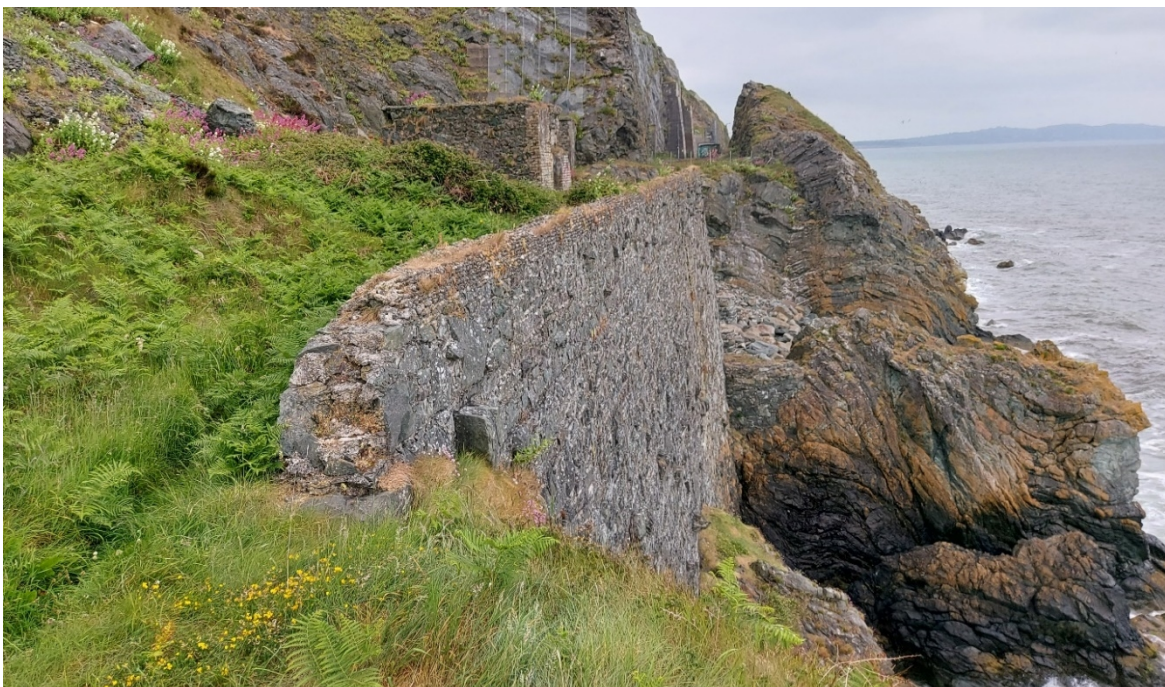
Figure 2 – CCA5-A: In some locations, masonry retaining walls have been installed to support the railway; these also serve as a coastal defence. In this image, the wall is located between two outcrops. In the upper section of the image, rock netting can also be seen, protecting the railway from debris and rockfalls.
