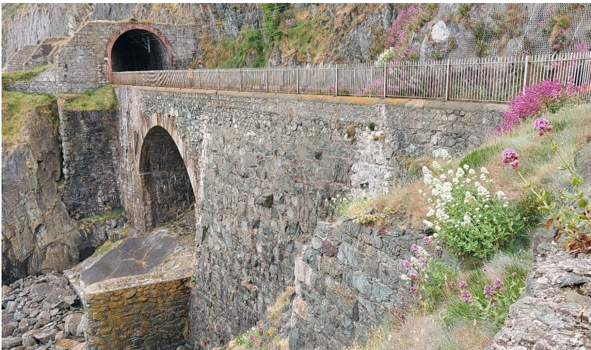
Figure 4 – CCA5-A: The railway within this sub-cell also goes through 4 tunnels, providing both coastal and rock fall protection. In this image, the entrance of Tunnel 1 is visible. A stone bridge/wall is located above the water level, and large boulders are located at the bottom of the asset.
