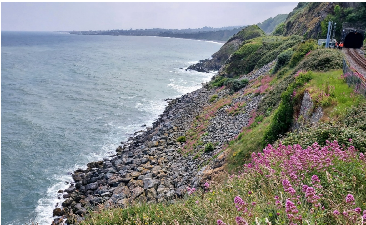
Figure 5 – CCA5-A: The entrance to Tunnel 4 can be seen here, with a rock armour protecting the toe of the asset. The boulders are very large and provide efficient coastal protection. Vegetated slopes are present between the rock armour and the railway. A retaining wall is also present on the right-hand side.
