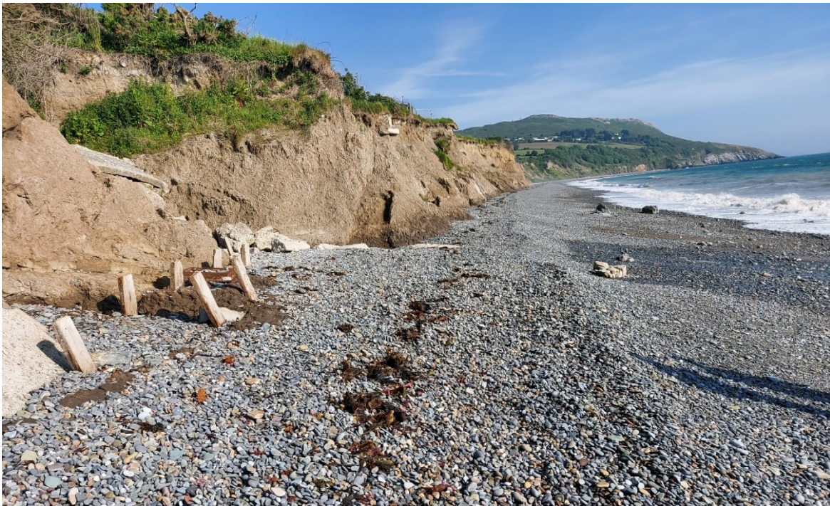
Figure 7 – CCA5-B: In the southern section of the beach, the cliff has suffered from significant erosion and subsequent landslides. The lack of vegetation highlights the steepness of the cliff and the recent erosion. The beach is also narrower, steeper and has a higher shingle content at this end of the beach.
