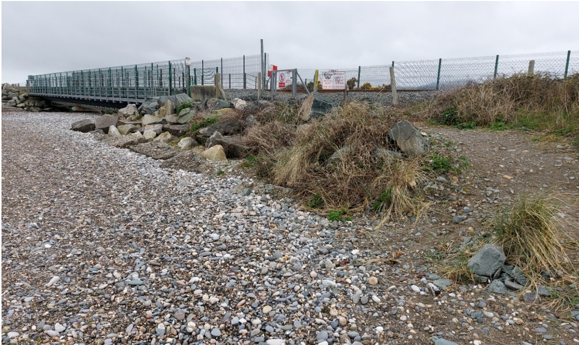
Figure 6 – CCA6.1-D: The separation between sub-cells CCA6.1-D and CCA6.1-E is located at Kilcoole Estuary, also known as 'The Breaches'. The beach is very dynamic and the position of the estuary channel is known to fluctuate. The railway crosses the estuary over a bridge, the abutments are protected from erosion by boulders.
