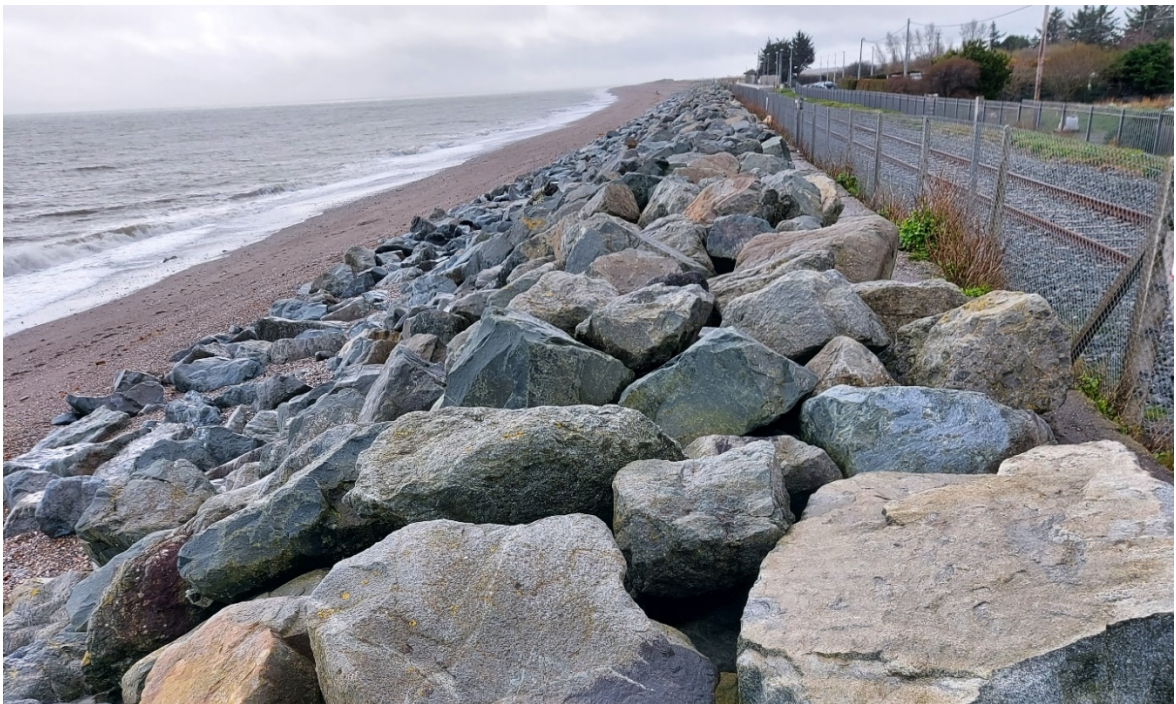
Figure 4 – CCA6.1-C: The sub-cell is a 1.8 km long section with rock revetment and concrete blocks at the back, located at the front of Kilcoole station. A relatively narrow and steep shingle beach is present in front of the revetment.
