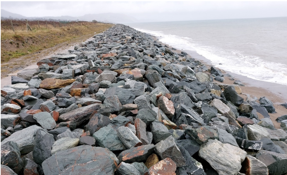
Figure 3 – CCA6.1-B: The rest of the sub-cell is also protected by a rock revetment and concrete blocks at the back. In this section, the rock used is of a smaller grading and is regularly displaced by wave action. The clearance between the sea and the track is large here, providing some additional protection to the railway.
