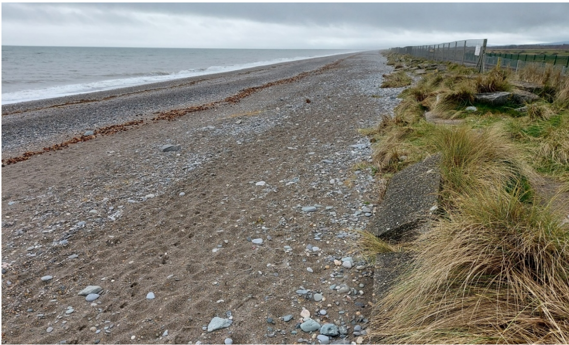
Figure 7 – CCA6.1-E: The rest of the cell is protected by a 40m wide sand and shingle beach, located between Kilcoole Estuary and Newcastle Airport. At the back of the beach, a narrow strip of vegetation is present with concrete blocks interspersed throughout. Beach levels remain stable in this area.
