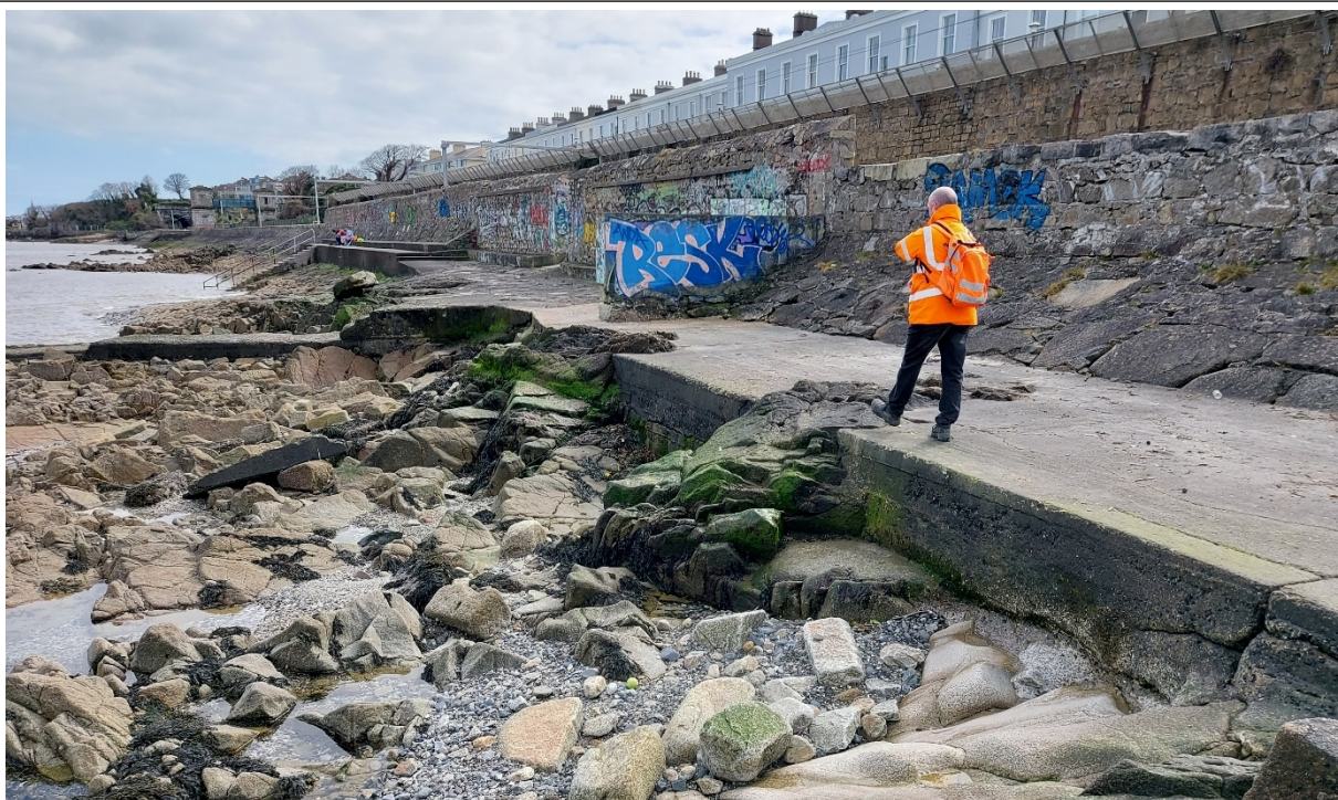
Figure 6 - CCA1-D: The sub-cell's defended section is protected by a masonry revetment and an upstand wall. A concrete walkway has been added along the defences. The foreshore is mainly rocky.
