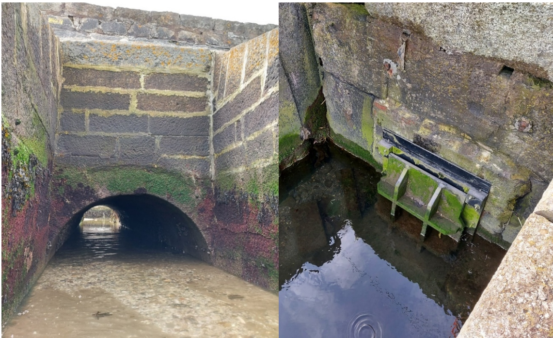
Figure 2 - CCA1-A: A stream located behind the railway and the existing surface water network which discharges to the sea through a series of culverts crossing the revetment. Some of these culverts include a flap gate to prevent upstream flooding during high tide.
