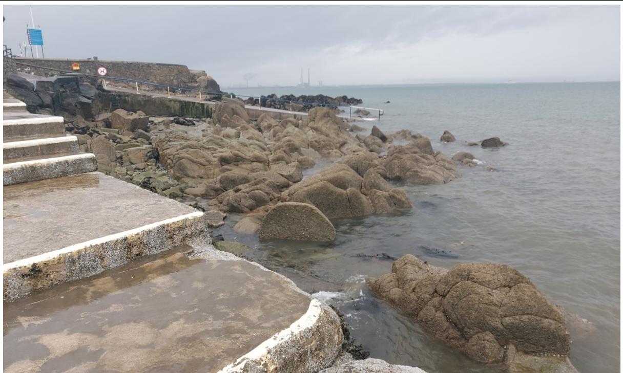
Figure 10 - CCA1-E: At the west of the sub-cell, there is a rocky outcrop with a Martello tower and a concrete walkway. There are several sets of steps and ramps providing access to the Seapoint Beach bathing area. The foreshore is rocky.
