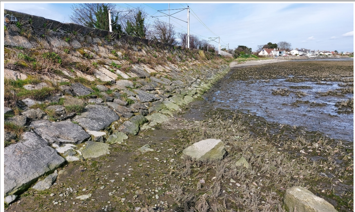
Figure 1 - CCA1-A: The sub-cell defence consists of a masonry revetment and an upstand wall. The northern half of the sub-cell is protected by a vegetated sand beach, while the southern half has muddy/marshy foreshore which is covered at high tide.
