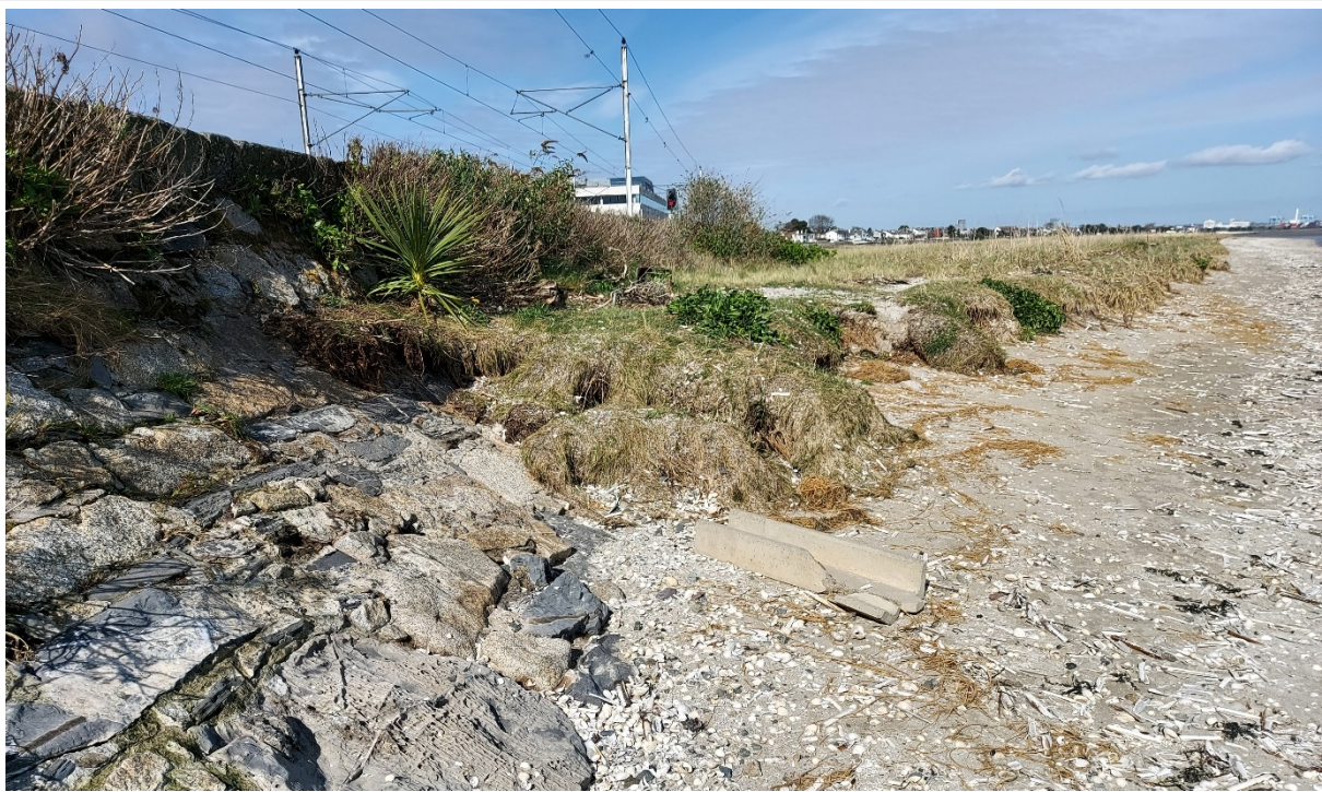
Figure 3 - CCA1-B: The sub-cell's engineered section is very similar to CCA1-A, with a masonry revetment and upstand wall close to the railway. In recent years, a sand spit has been accumulating in this area, providing additional coastal protection and habitat for birds.
