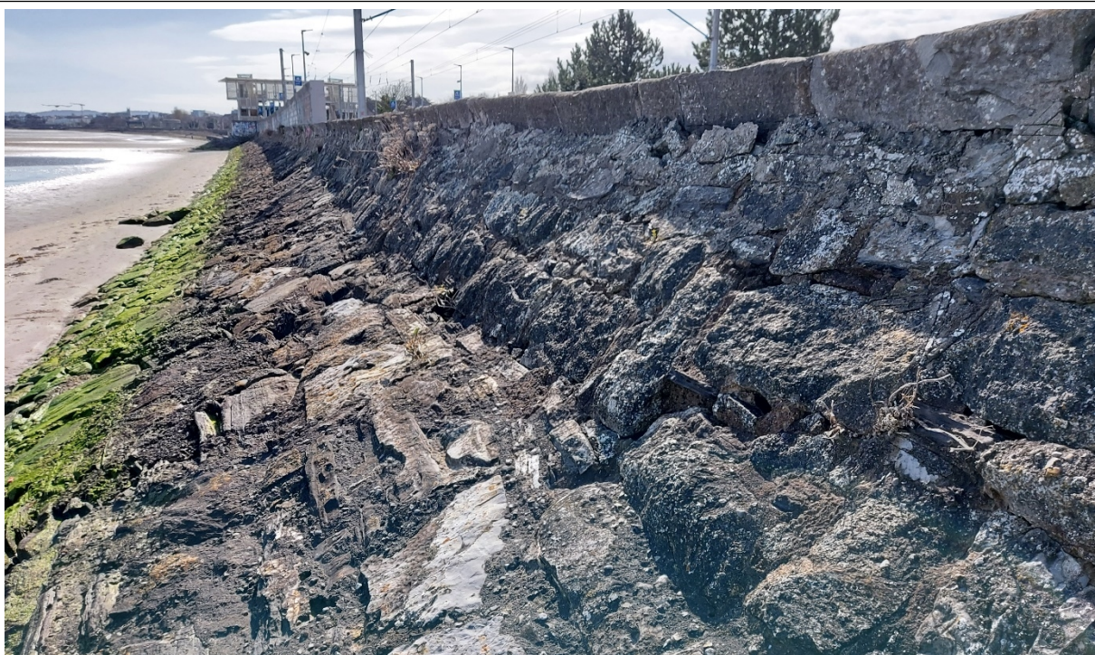
Figure 4 - CCA1-C: The sub-cell consists of a masonry revetment and an upstand wall. The area also includes Booterstown station, where an additional wall upstand has been added in recent years. The foreshore is sandy/silty and fully covered at high tide; algae are visible along the bottom of the defence.
