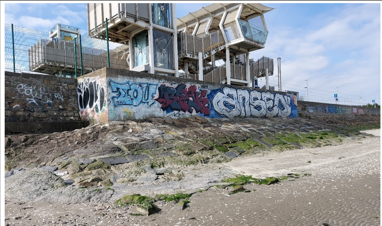
Figure 5 - CCA1-C: Booterstown station's coastal protection is very similar to the rest of the sub-cell, but with a higher upstand wall which protects the public from sea spray. The station is under additional pressure from storm events due to extending further onto the foreshore.
