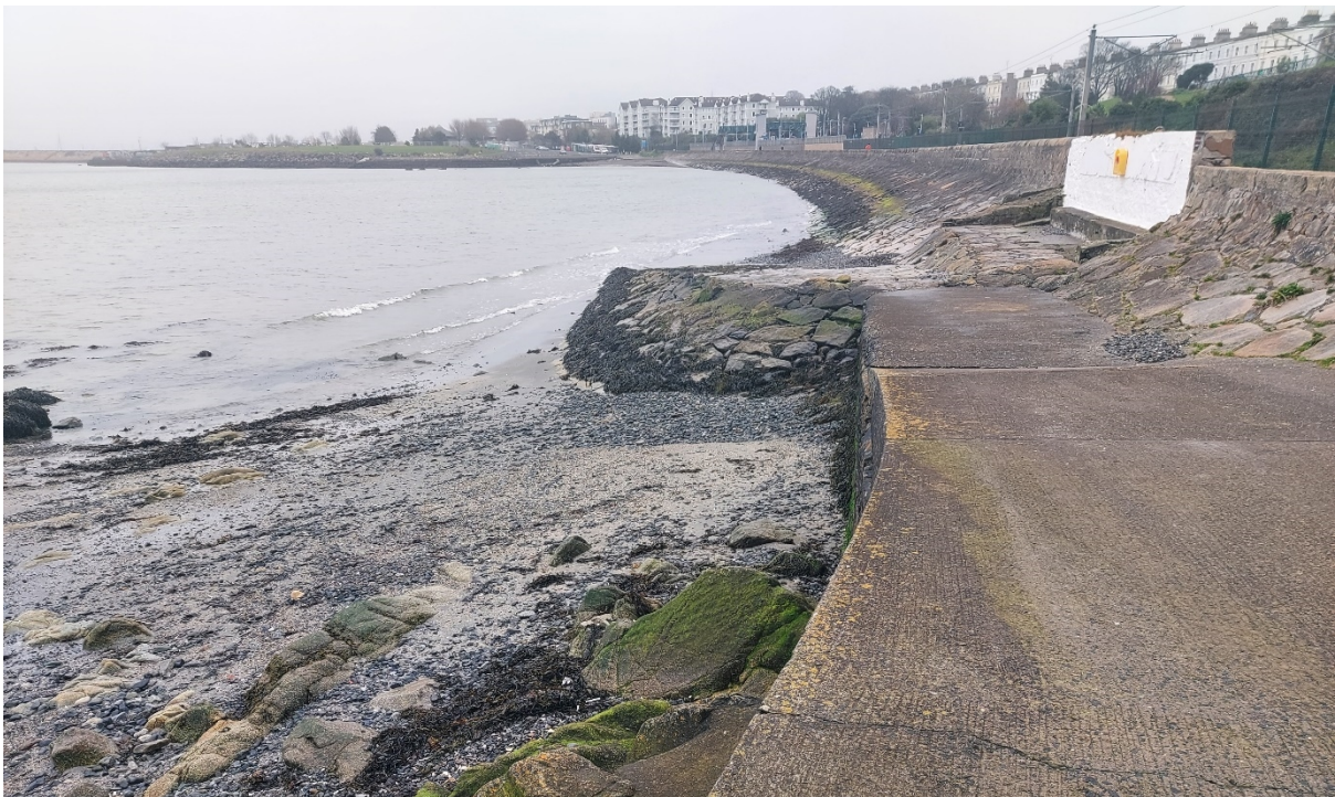
Figure 12 - CCA1-E: Throughout the sub-cell, the defence is a sloping masonry revetment with upstand wall. A walkway runs along parts of the sub-cell, with a short gravelly beach. There is no foreshore at high tide in the eastern half of this cell.
