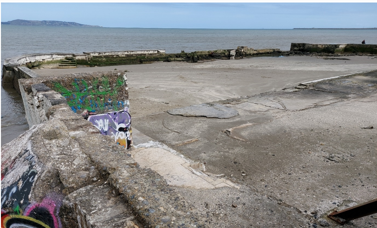
Figure 7 - CCA1-D: Historic baths are located within the northern part of the sub-cell, which are now disused. The remains of the baths are currently providing additional coastal protection, but a masonry revetment and upstand wall are located in front of the railway.
