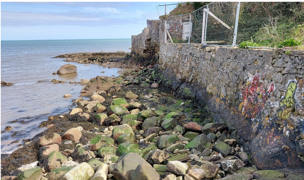
Figure 8 - CCA1-D: In the centre of the sub-cell, a small rocky headland with rocky foreshore is present and provides natural protection to the railway. A masonry wall is present along much of the headland.
