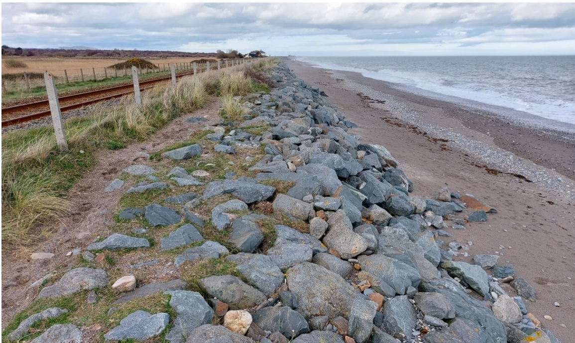
Figure 2 – CCA6.2-A: The second half of the sub-cell is protected by a 20m wide sand and shingle mix beach. At the back of the beach, there is some rock scour protection; the upper portion of the scour protection is vegetated. Evidence of localised erosion is visible.
