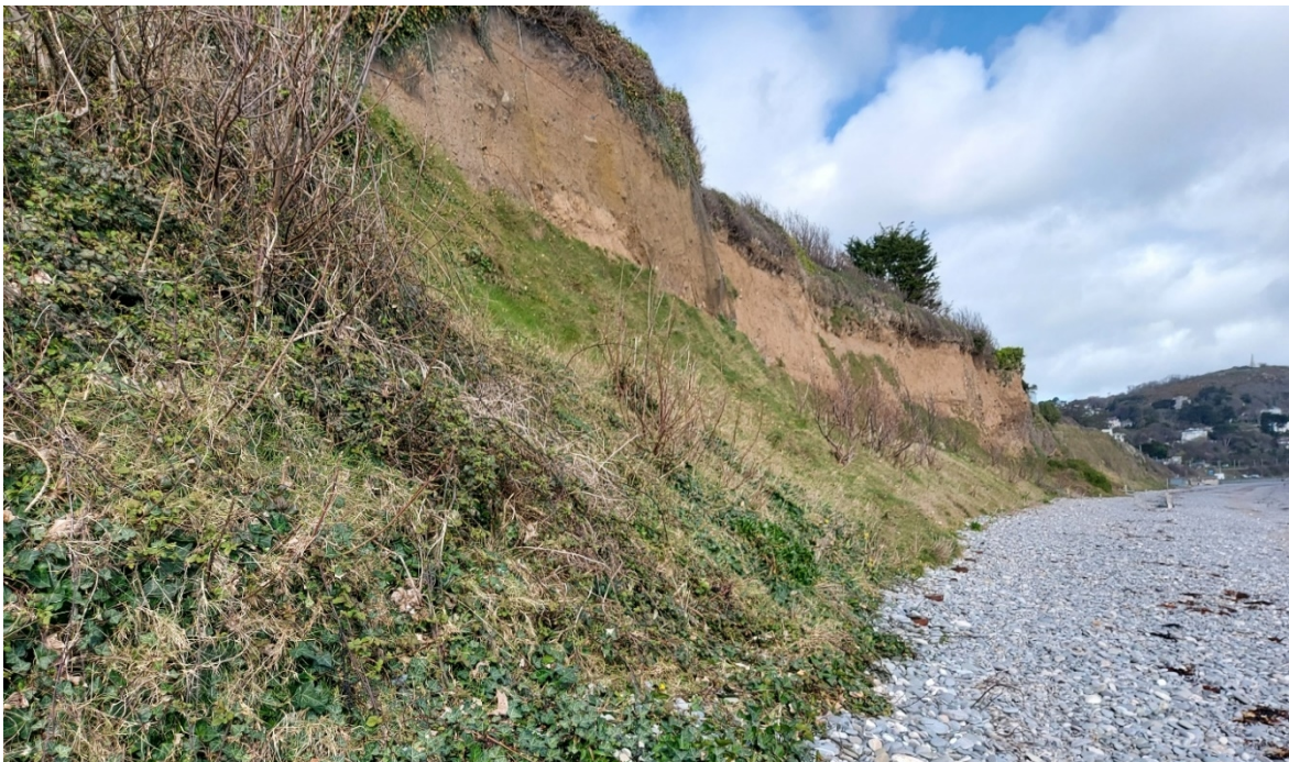
Figure 8 – CCA2/3-D: The sub-cell is in front of several properties which are located between the beach and the railway. The soft cliffs here have suffered from erosion with failures of the slope toe. Vegetation has covered the slip, but uncovered cliff faces can still be seen. The beach is made of the same coarse material.
