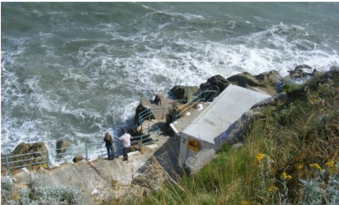
Figure 2 – CCA2/3-A: Vico baths are a series of concrete steps located at the bottom of a rock outcrop, popular for sea bathing. The railway is protected by this natural outcrop and the presence of large boulders in the foreshore.
