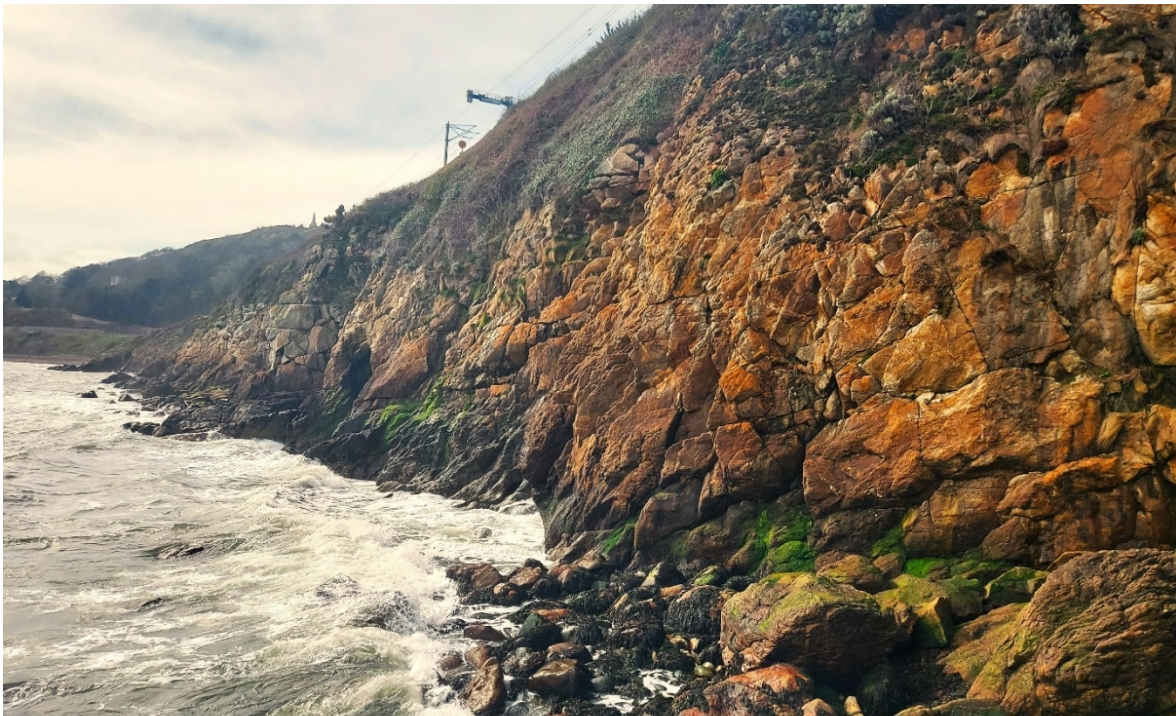
Figure 3 – CCA2/3-A: The rest of the sub-cell is made of a natural rock face, with a varying cliff height of approximately 40 meters. Rocks which have fallen now make the foreshore and provide additional coastal protection. The upper part of the cliff is stabilised by vegetation.
